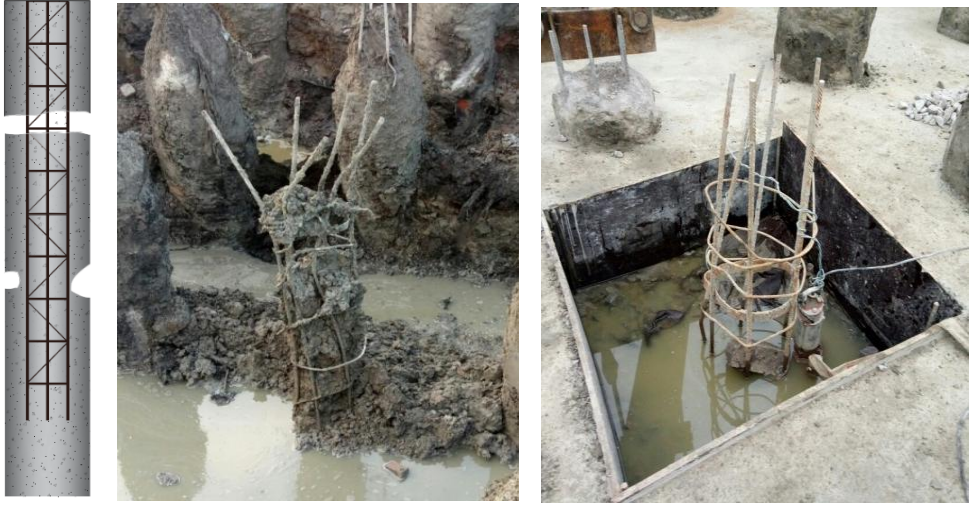
Figure 3 – Washout of concrete mixture
